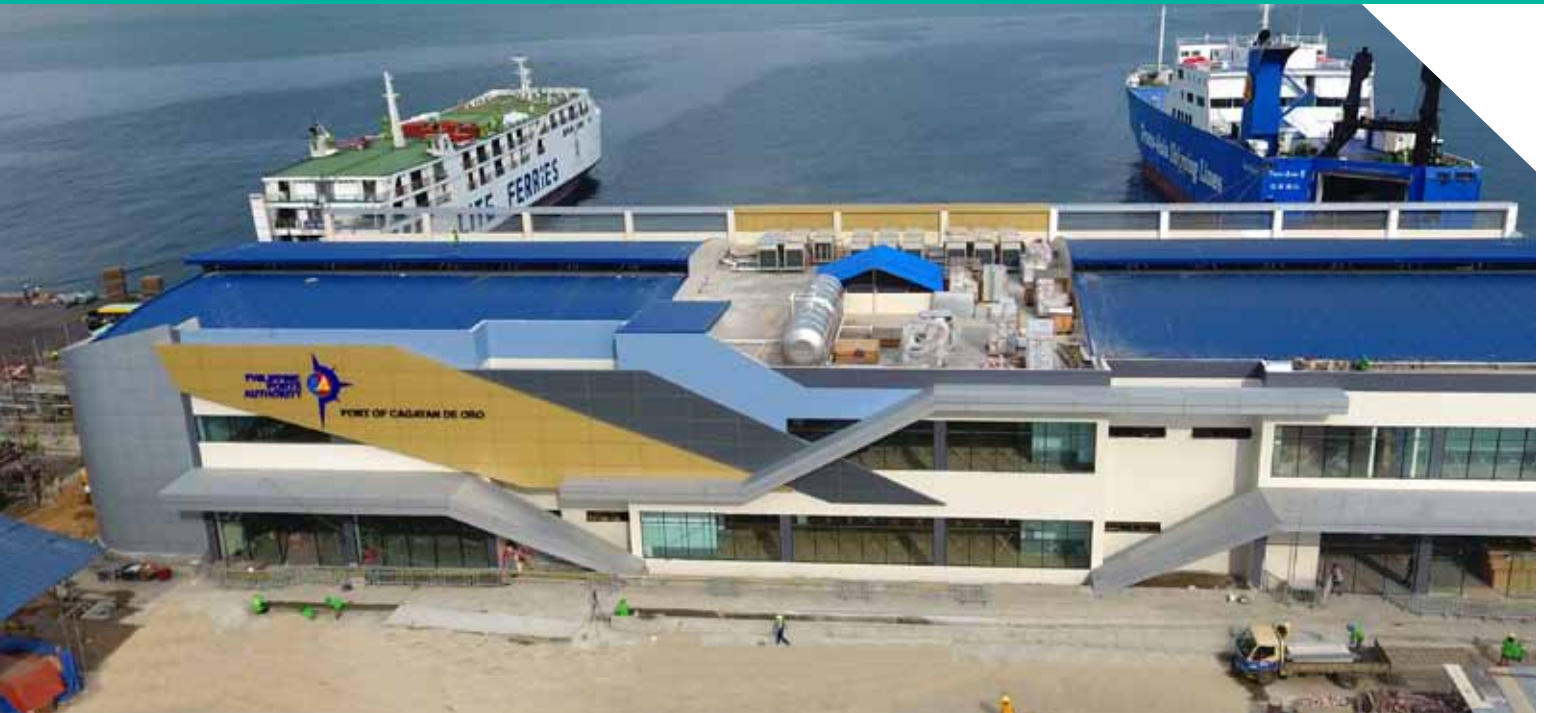
Above: By July 2019, the country's biggest passenger terminal will open its doors. The new PTB at the Port of Cagayan de Oro will showcase modern port facilities, including x-ray scanning machines, walk-through metal detectors, among others. The PTB complex will soon be able to cater to over 3,000 passengers daily.
